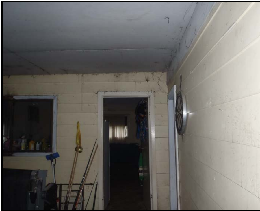
Photo 17: 12 Horton Road (residence): Photo showing the ACM panelling present within and ACM sheeting used in the ceiling lining to the extension.
