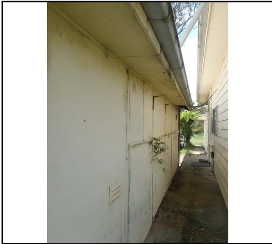
Photo 7: 14 Horton Road: A section of the southern wall to the garage lined with ACM sheeting.
