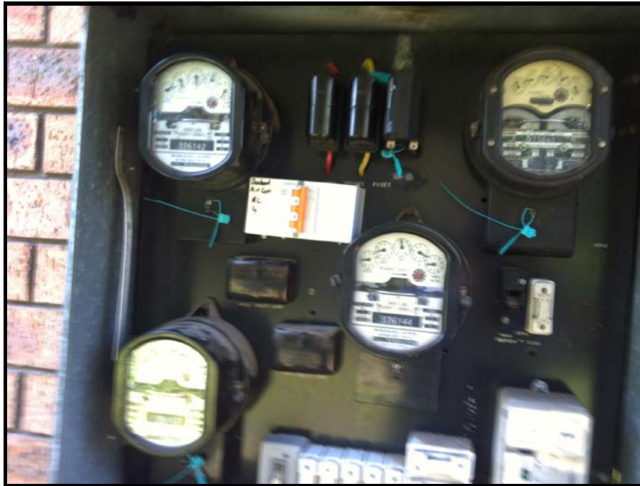
Photo 23: Scales Avenue: The zelemite backing board to the electrical switchboard.
