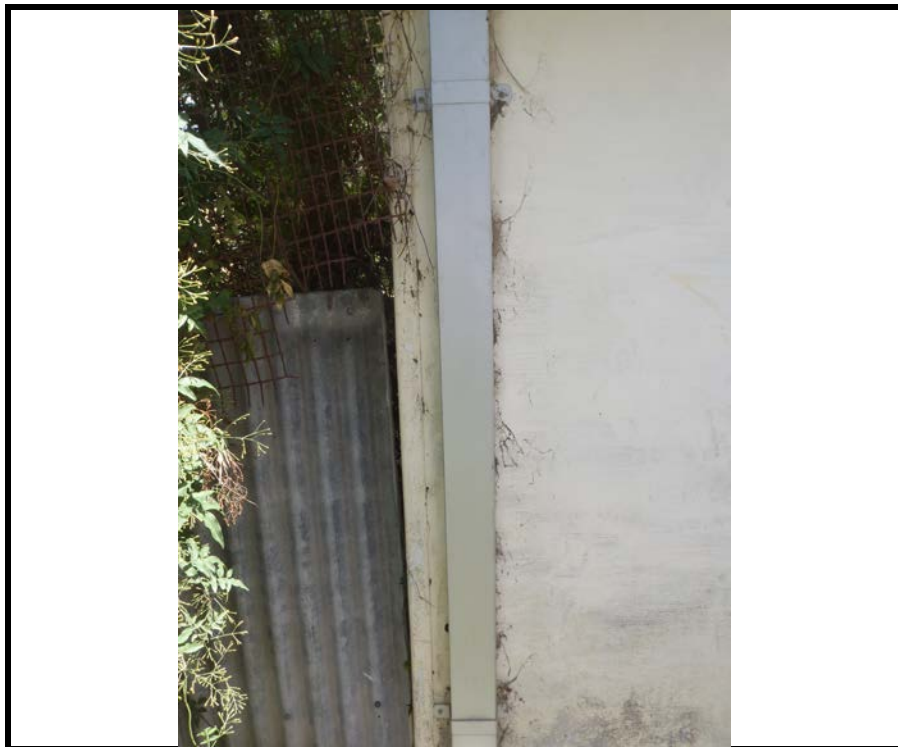
Photo 8: 14 Horton Road: the corner moulding to the southwest corner to the garage comprised of ACM
