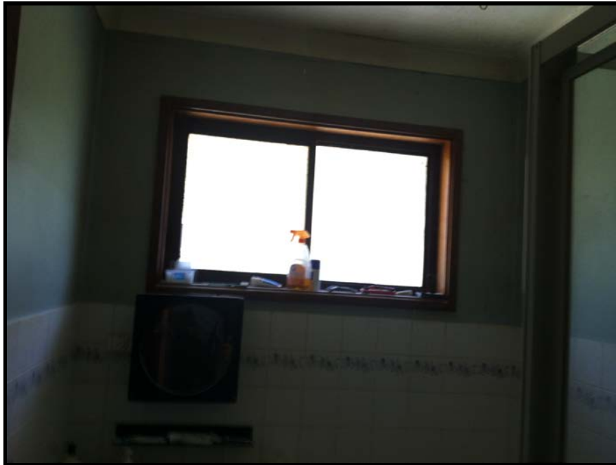
Photo 21: Scales Avenue: The bathroom with walls lined with ACM sheeting.
