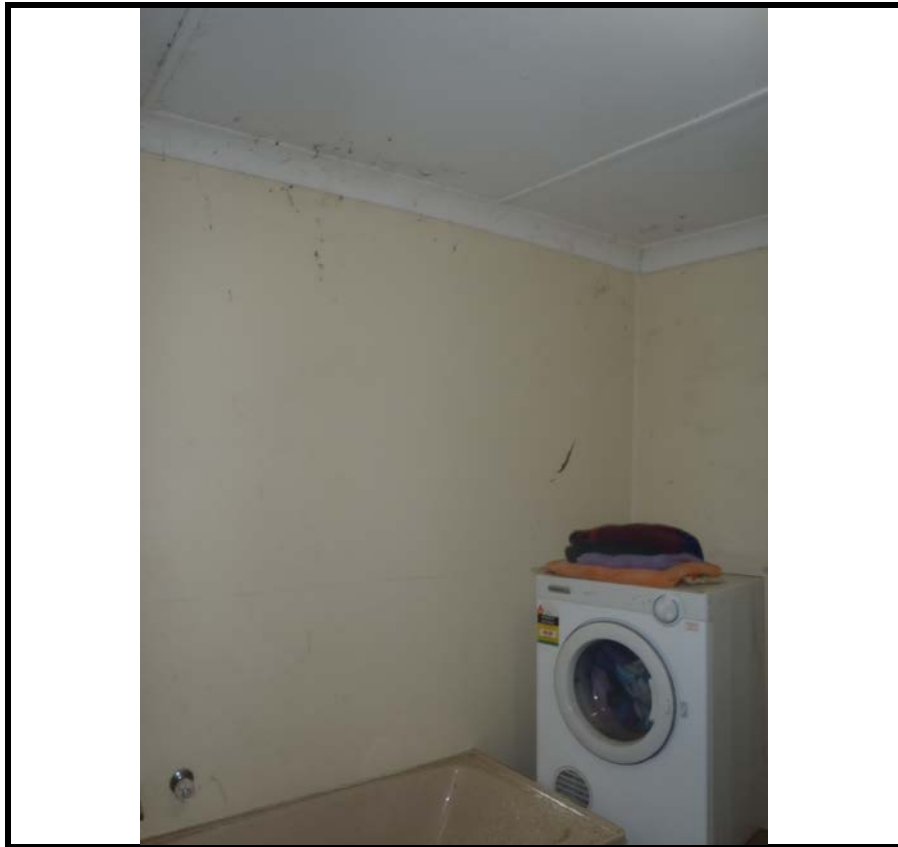
Photo 19: 12 Horton Road (residence): A section of the laundry/ bathroom with the walls and ceiling lined with ACM sheeting.
