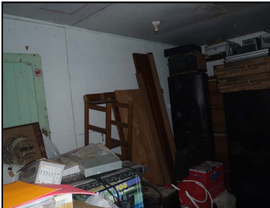
Photo10: 14 Horton Road: An example of ACM sheeting lining the walls in the rear of the garage. Other sections have been wallpapered.
