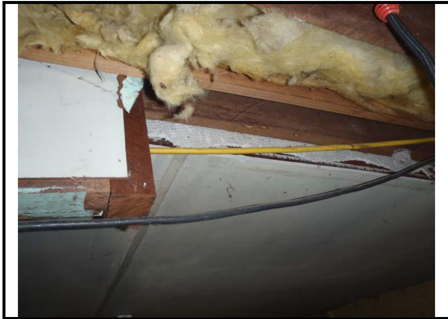
Photo 11: 14 Horton Road: This photo in the garage shows some of the exposed SMF, a section of broken ACM sheeting attached to the beam, and ACM sheeting used to line the ceiling.
