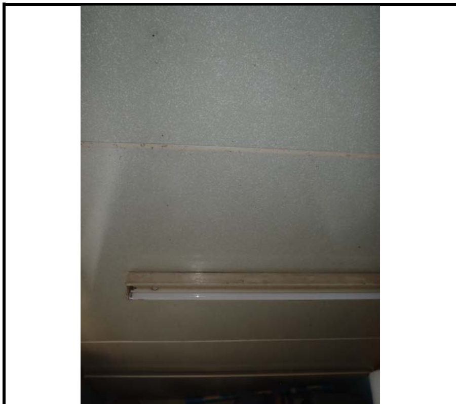
Photo 2: 14 Horton Road: An example of one of the interior fluorescent lights that may have a PCB-containing capacitor.
