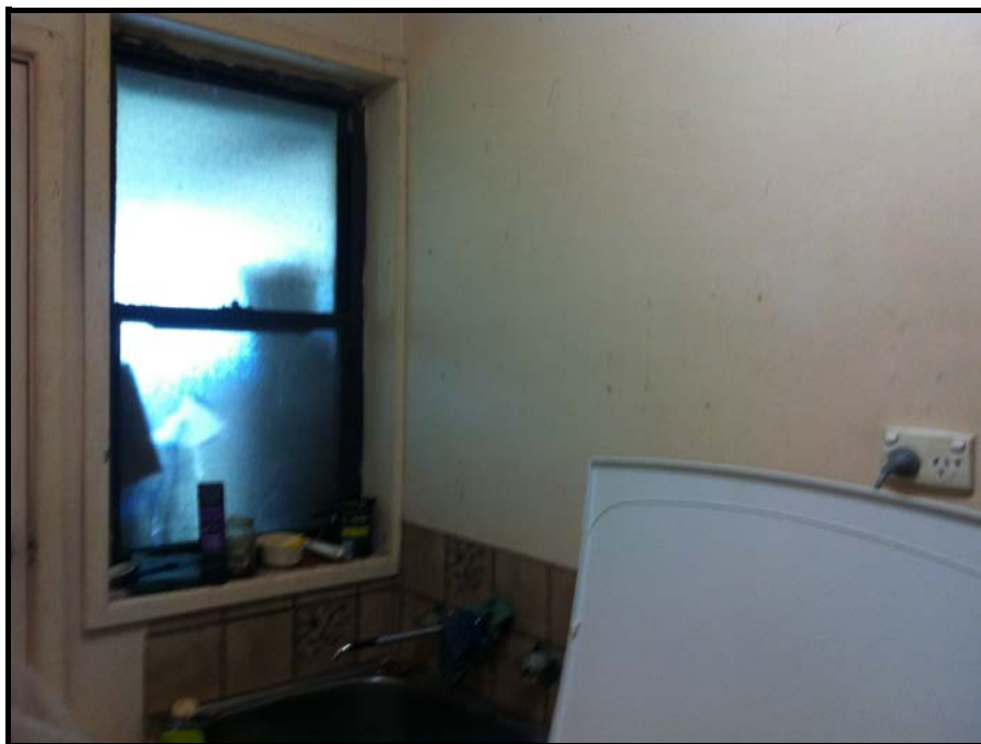
Photo 22: Scales Avenue: The laundry with walls and ceiling lined with ACM sheeting.
