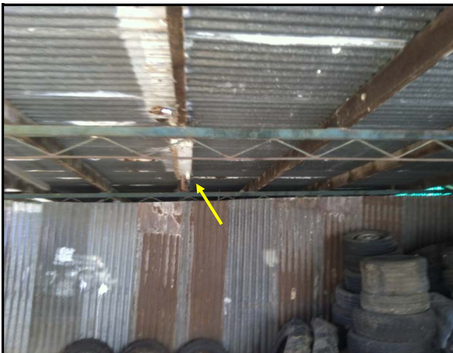
Photo 26: 12 Horton Road (Business): Fluorescent light fitted to metal frame in carport to small shed
