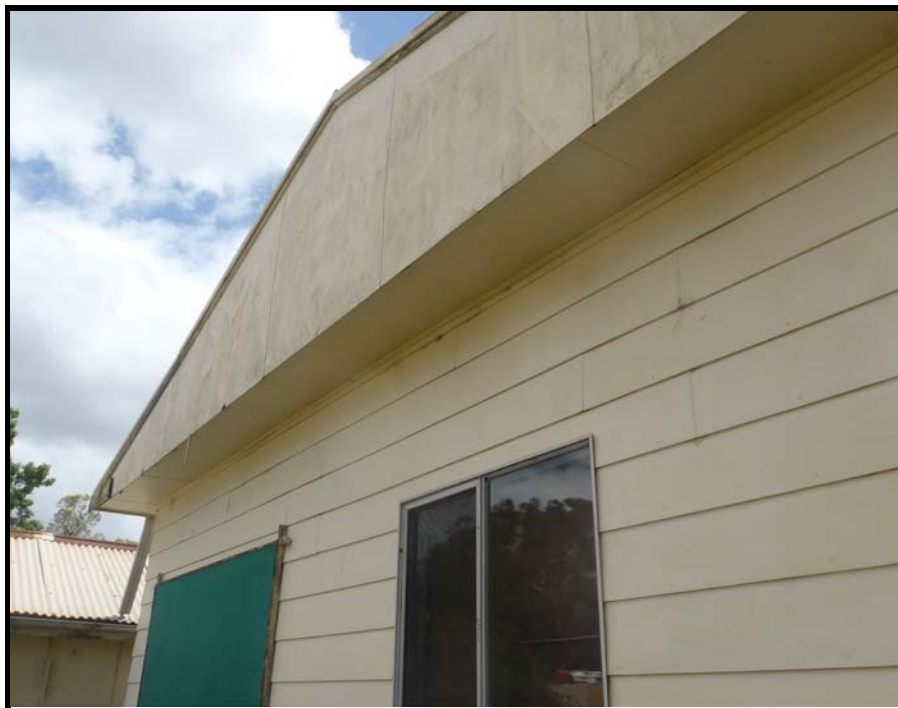
Photo 4: 14 Horton Road: An example of the eaves and one of the gable ends assumed to be constructed of ACM sheeting.
